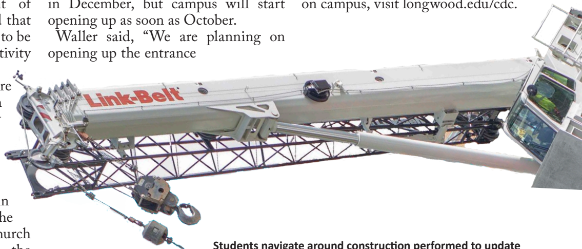
Students navigate around construction performed to update the steam tunnels running throughout campus, a project that is estimated to be completed late December, early January
