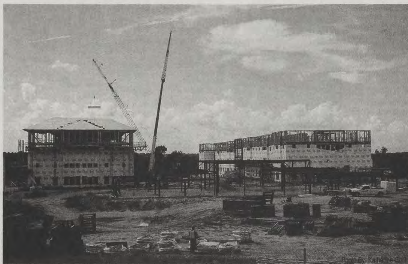
The North Campus construction is well underway at Lancer Park. The completion date is currently set to be in June of 2013.
