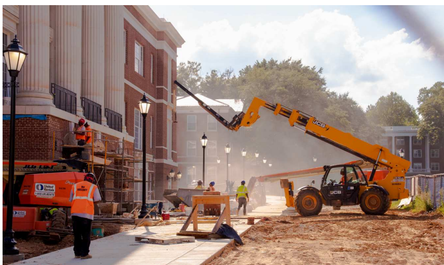
Construction workers add the finer details into the back entrance of the Upchurch Center.
