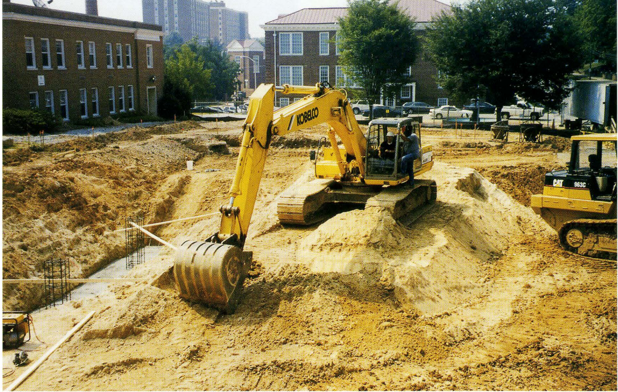
Dr. Patricia P. Cormier, donning a hard hat and perched inside a backhoe, scooped out a ceremonial shovelful of dirt.
