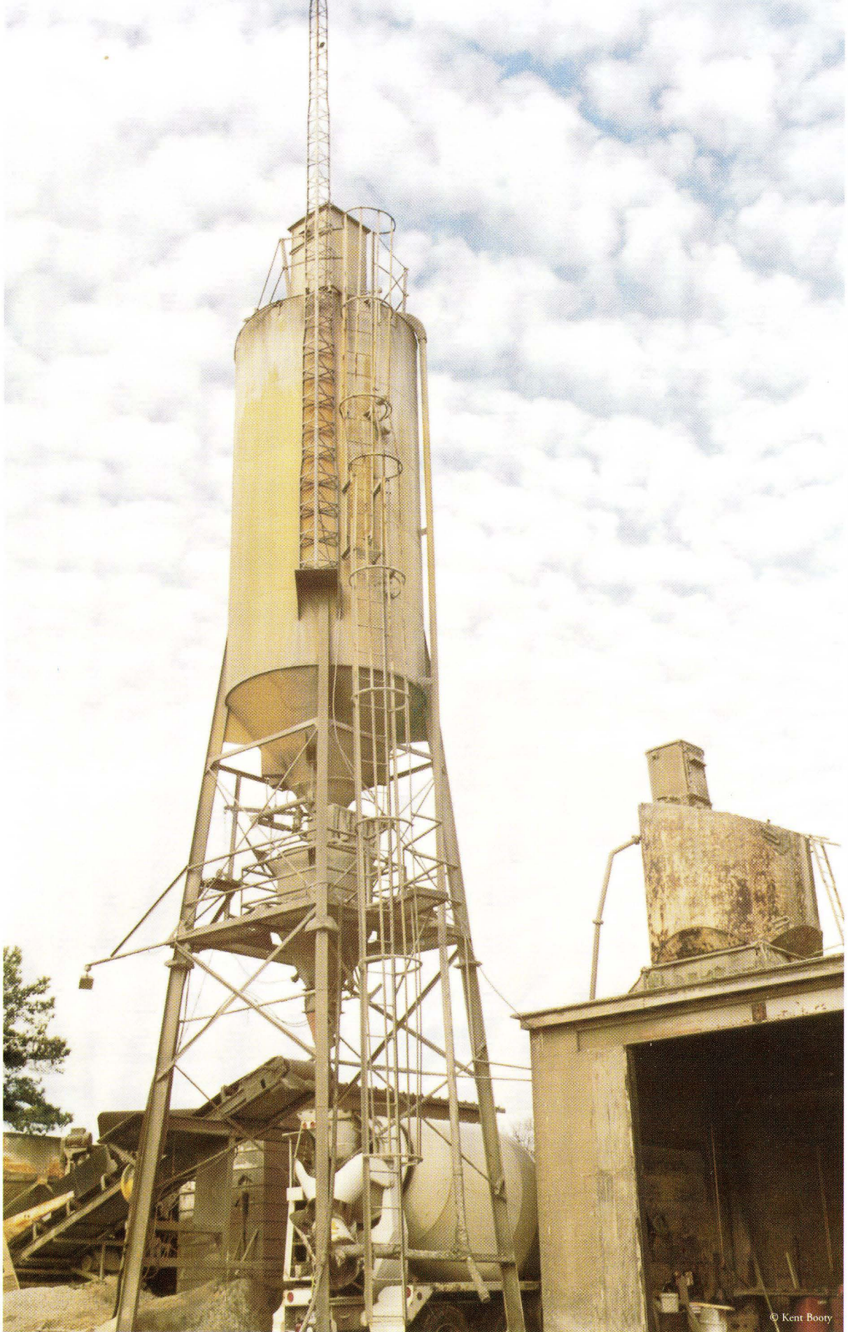
The yellow silo, just behind the office, can hold three tanker loads of bulk cement. The tanker usually delivers 55,000 pounds.
